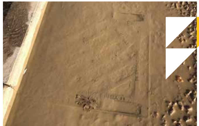
Ironwork after being exposed to typical construction site traffic.
